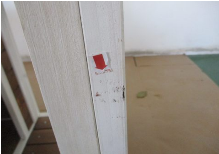
Minor defect: paint stain
