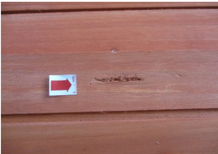
Minor defect: chipped on bottom board
