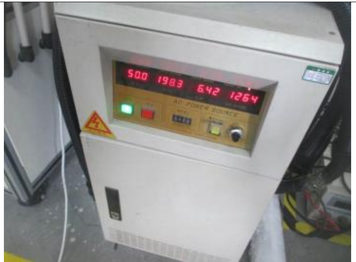
Low voltage starting check
