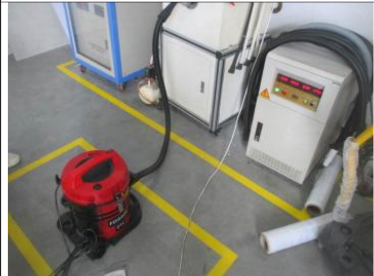
Low voltage starting check
